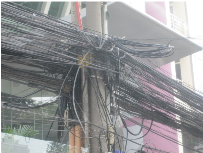
An Electrician's Nightmare
